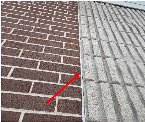
Photograph No. 29 Asbestos-Containing grey expansion caulking (Sample Group 25017022-ASB-19A-C). Exterior wall.
