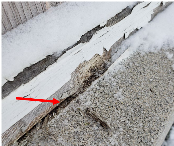
Photograph No. 31 Asbestos-Containing grey caulking (Sample Group 25017022-ASB-31A-C). Exterior windowsills.
