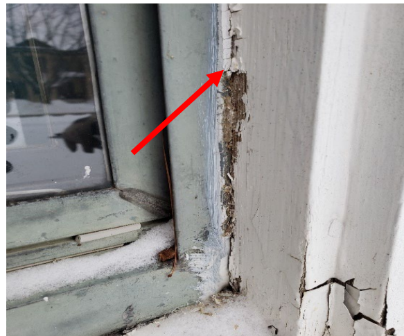
Photograph No. 32 Asbestos-Containing old white caulking (Sample Group 25017022-ASB-33A-C). Exterior windowsills.
