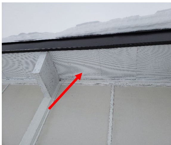
Photograph No. 10 Asbestos-Containing Transite boards. Exterior.
