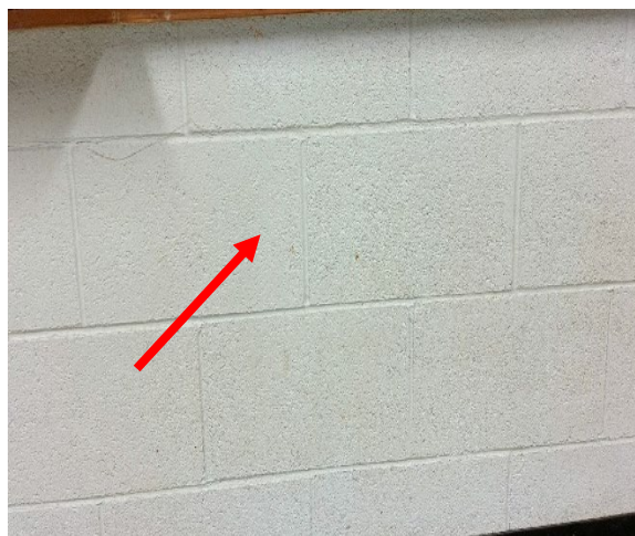
Photograph No. 9 Asbestos-containing concrete block filler compound concealed beneath paint on concrete block walls (Sample 25017022-ASB-02C).
