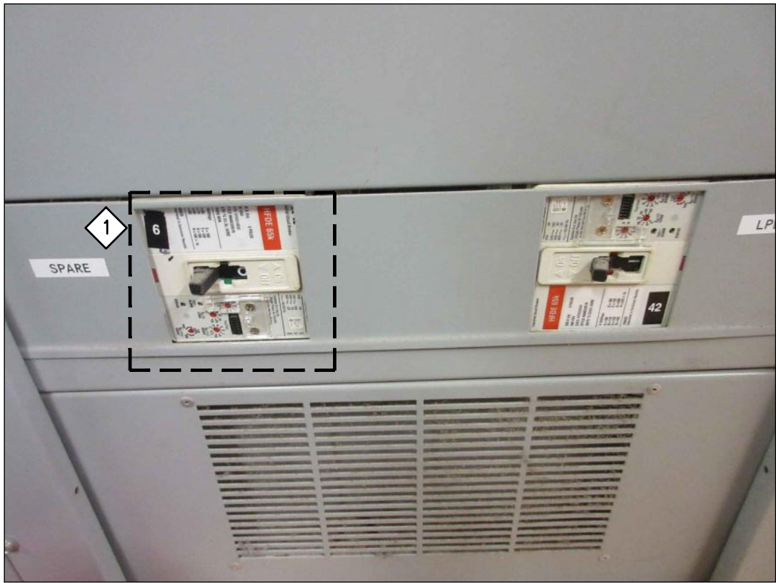
SPARE CIRCUIT BREAKER 06
