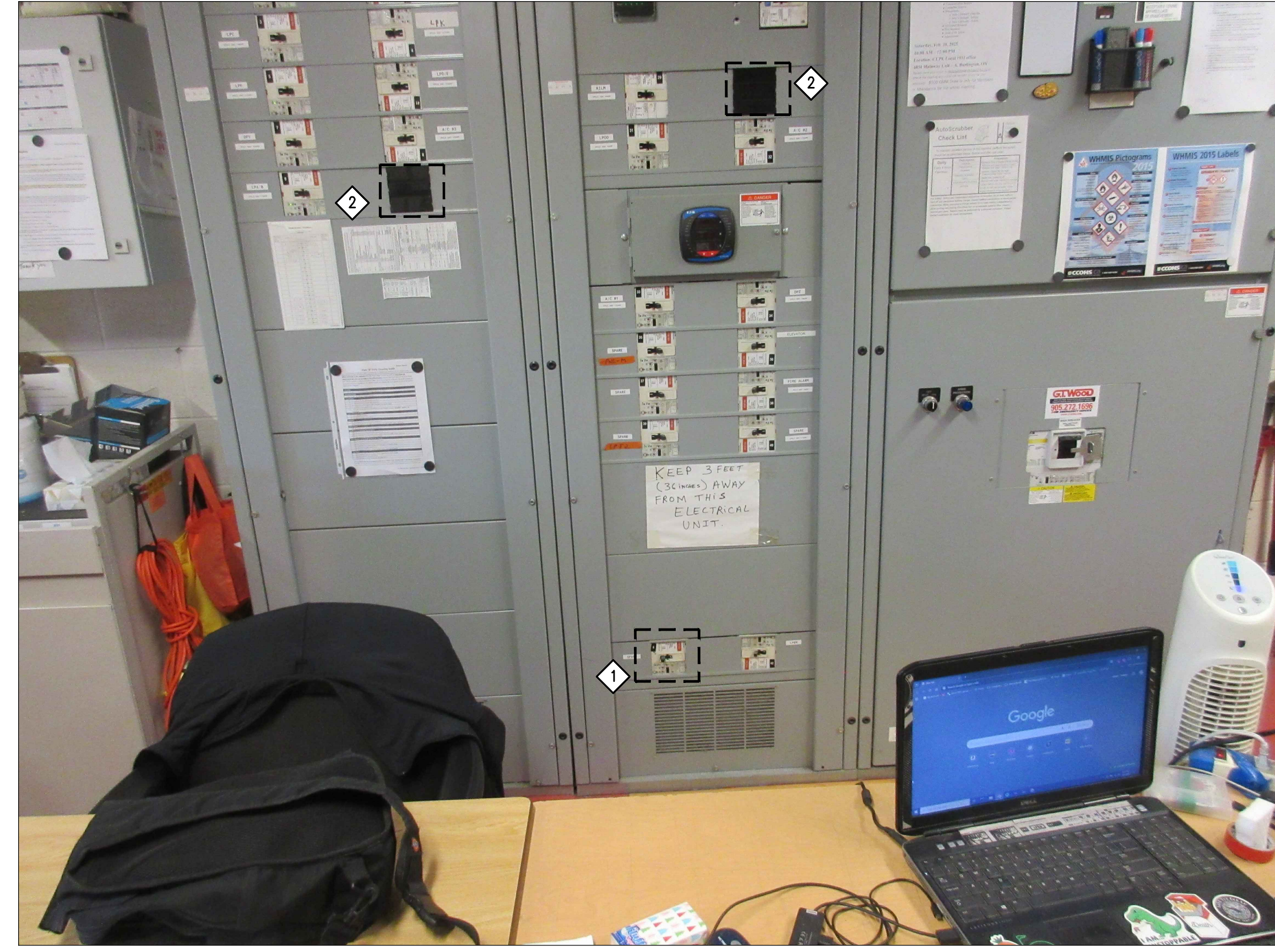
EXISTING MAIN SWITCHBOARD 'DP-Z' SCALE
