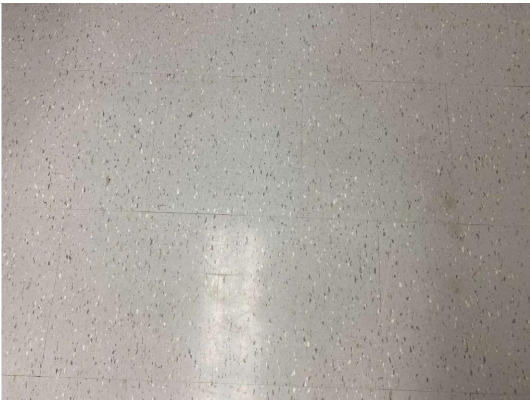
V0000 (None), 12x12 grey with white and dark grey fleck, Floor, Vinyl Floor Tile and Mastic, 1997 Addition First Floor (Location #: 1)
