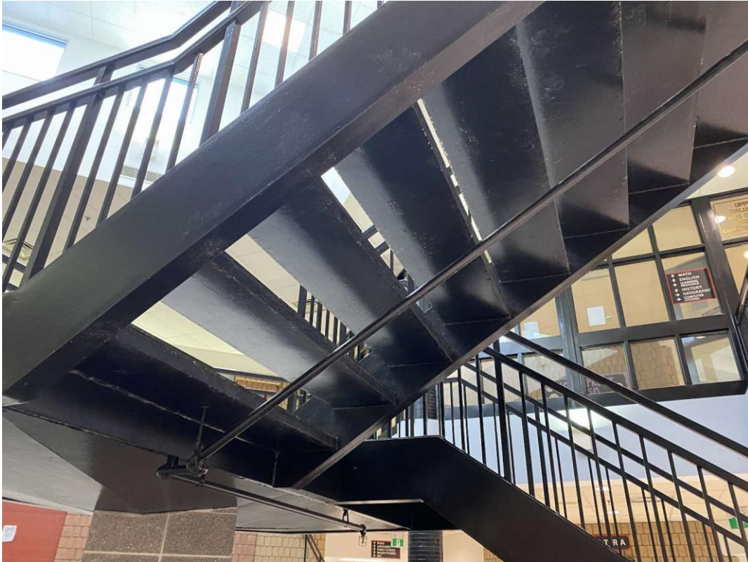
L0002(Lead, None), Black stairwell, Other, Learning Commons / Atrium / Foyer / Study Rooms (Location #: 4)
