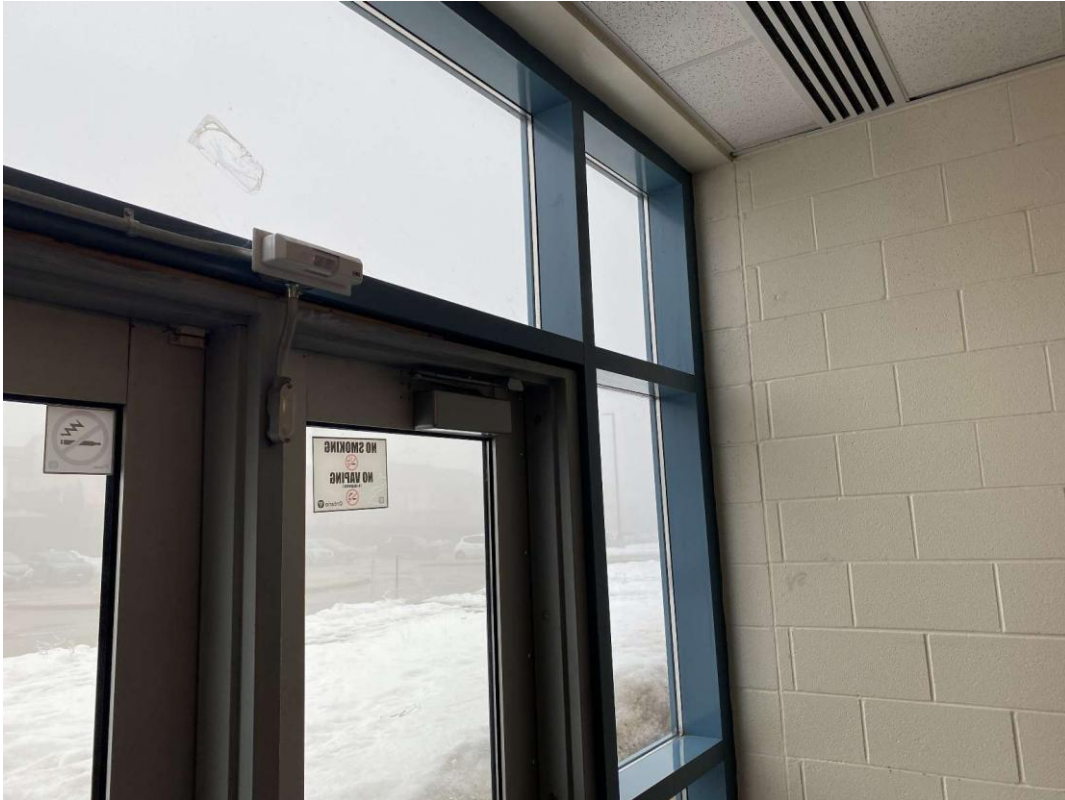
S0008A (None), Black, Other, Door, Caulking, Stairwell K1 Doors (Location #: 9)
