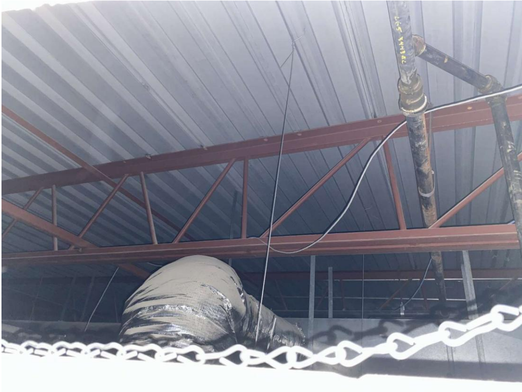
V9500(Presumed Lead), Red primer, Structure, Washrooms and Custodial Area (Location #: 16)
