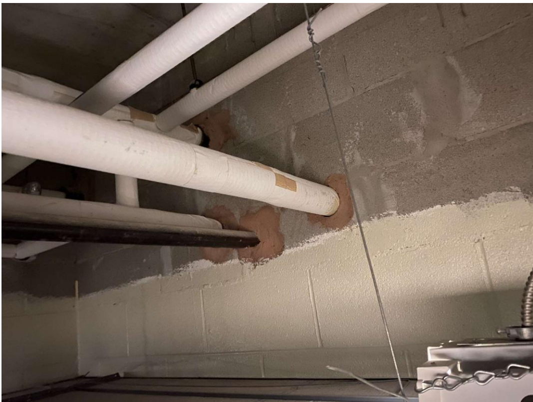
S0007A (None), Other, Firestopping (Cementitious), Girl's Washroom (Location #: 20)
