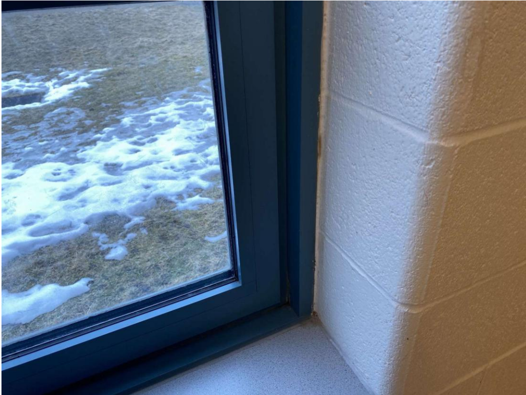
S0003A (None), White, Other, Window, Caulking, 1997 Addition First Floor (Location #: 1)
