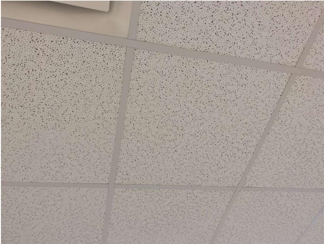
V0000 (None), 24x24 pinhole with fleck, Ceiling, ACOUSTIC TILE, Ceiling Tiles (lay-in), Play Rooms / Co-op Education (Location #: 6)
