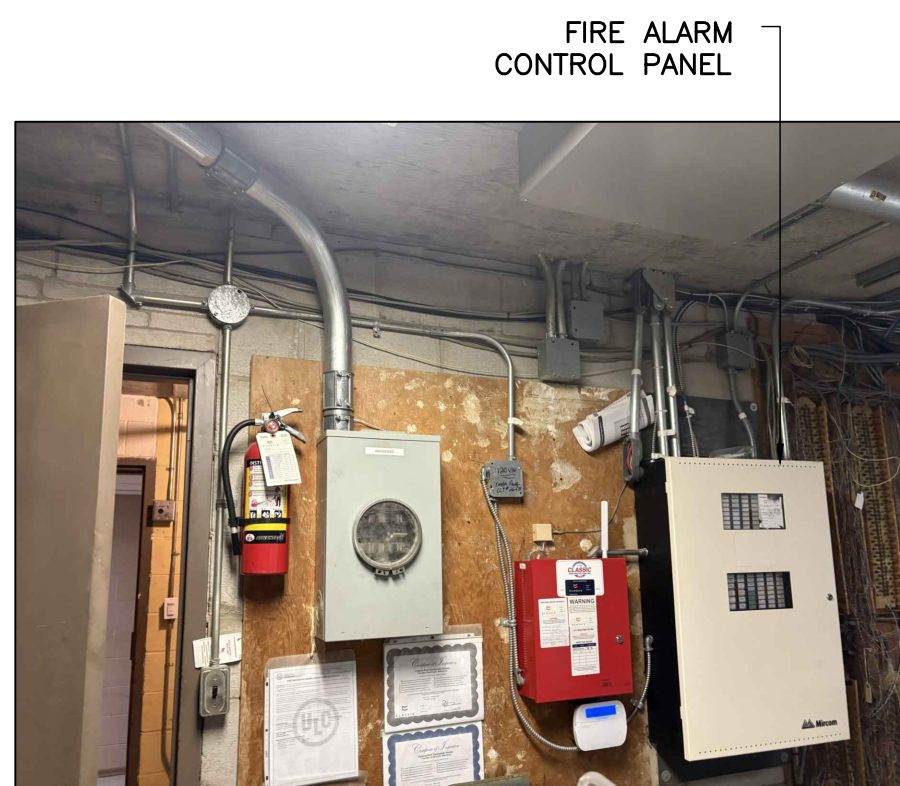
IMAGE 8 : EXISTING FIRE ALARM CONTROL PANEL(FACP)
