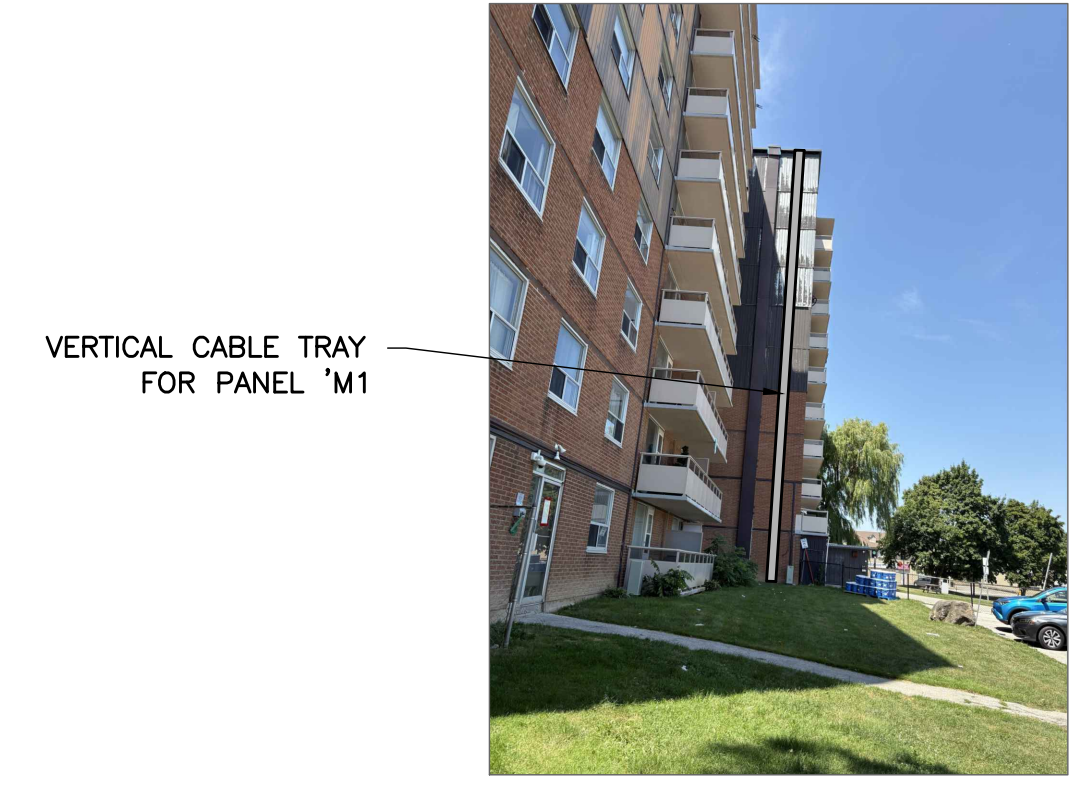
IMAGE 7: VERTICAL ELECTRICAL CABLE TRAY FOR PANEL M1
