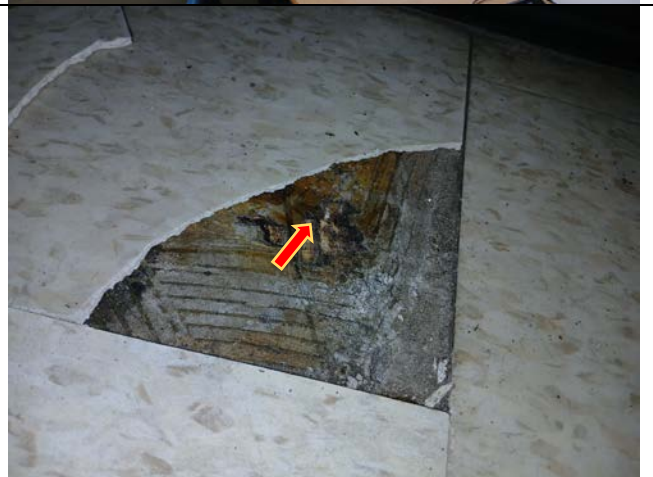
Photograph 5. View of asbestos-containing mastic identified under VFTs in Seminar Room 204 on the 2 nd floor at the Subject Location.
