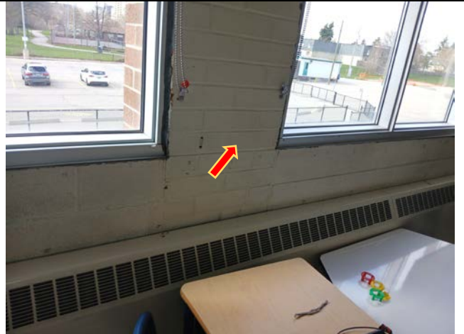
Photograph 4. View of the previously identified asbestos-containing interior brick mortar on the walls in Room 202 on the 2 nd floor at the Subject Location.
