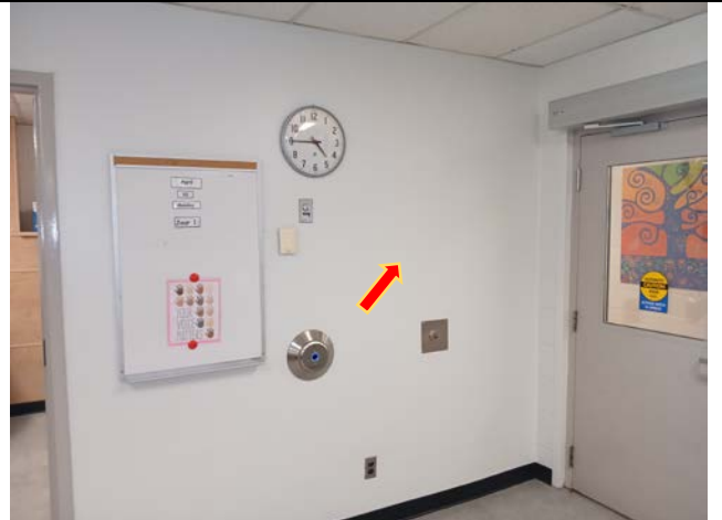
Photograph 1. View of the drywall with previously identified asbestos-containing DJC on the walls in General Room 137 on the 1 st floor at the Subject Location.
