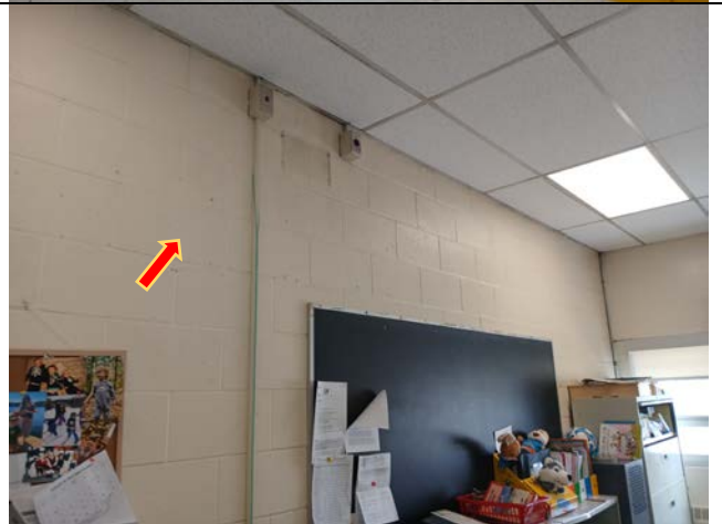
Photograph 3. View of the previously identified asbestos-containing primer on the walls in Work Room 203 on the 2 nd floor at the Subject Location.
