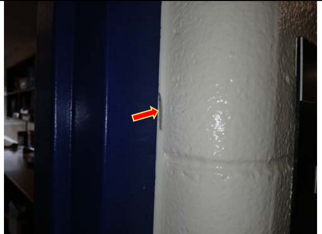
Photograph 7. View of asbestos-containing caulking identified around the door frame in Seminar Room 204 on the 2 nd floor at the Subject Location.
