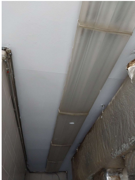
Photograph No. 12 – Mercury-containing fluorescent light tubes were observed throughout the interior. Associated light ballasts may contain PCBs.
