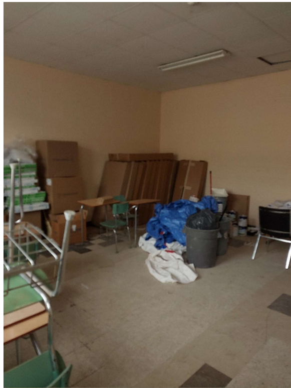
Photograph No. 14 – Beige paint was sampled from the walls of Room 1045 (LP01) and is low level lead-containing.
