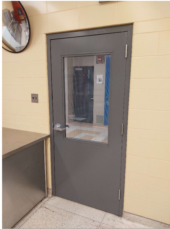
Photograph No. 16 – Dark grey paint was observed on doors to Room 1044 and was sampled (LP05). The paint is low level lead-containing.
