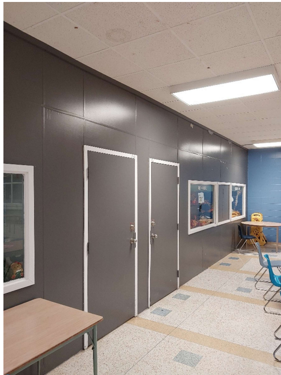
Photograph No. 8 – Drywall joint compound was observed on the interior of Rooms 1042A and 1042B. The compound was sampled (S07A,B,C) and is non-asbestos. The grey paint was sampled (LP04) and is low level lead-containing.
