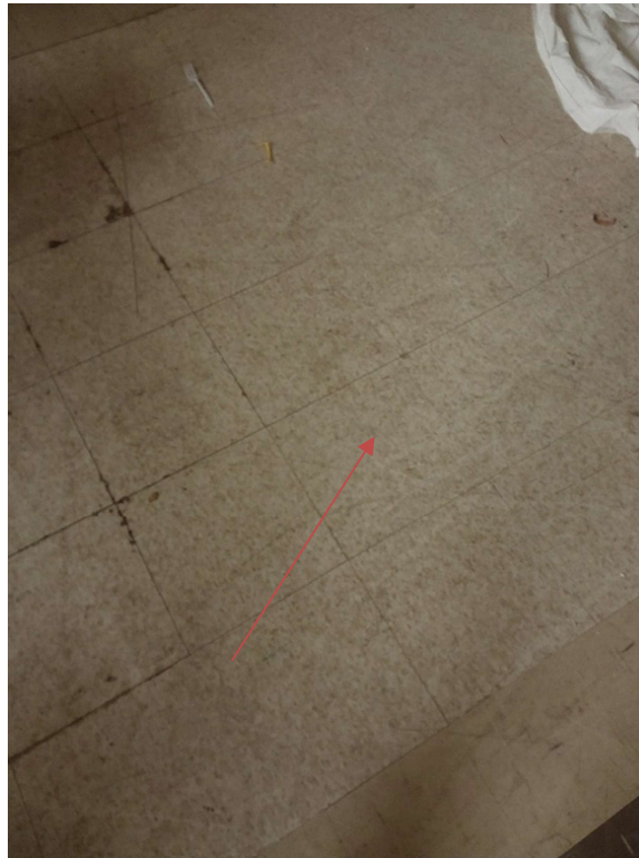
Photograph No. 5 – 12"x12" White with oat pattern vinyl floor tile was observed in Room 1045. The vinyl floor tile was sampled (S03A,B,C) and is non-asbestos; however, the associated mastic is asbestos-containing.
