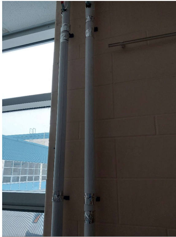
Photograph No. 11 – Fiberglass insulation with fiberglass elbows was observed in Room 1045 and does not contain asbestos.
