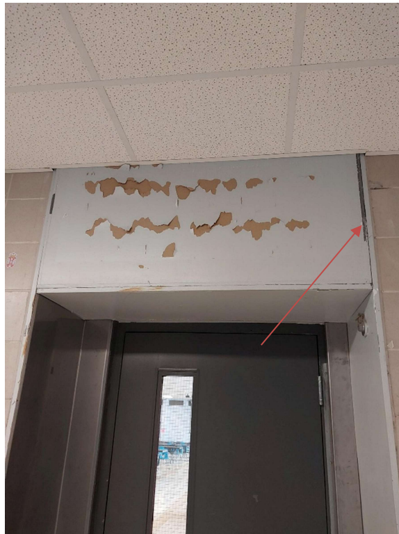
Photograph No. 19 – Drywall joint compound was observed on bulkheads above the doorway in Corridor 1043 leading into Room 1042. The compound was sampled (S10A,B,C) and does not contain asbestos. The light blue paint was also sampled (LP08) and is low level lead-containing.
