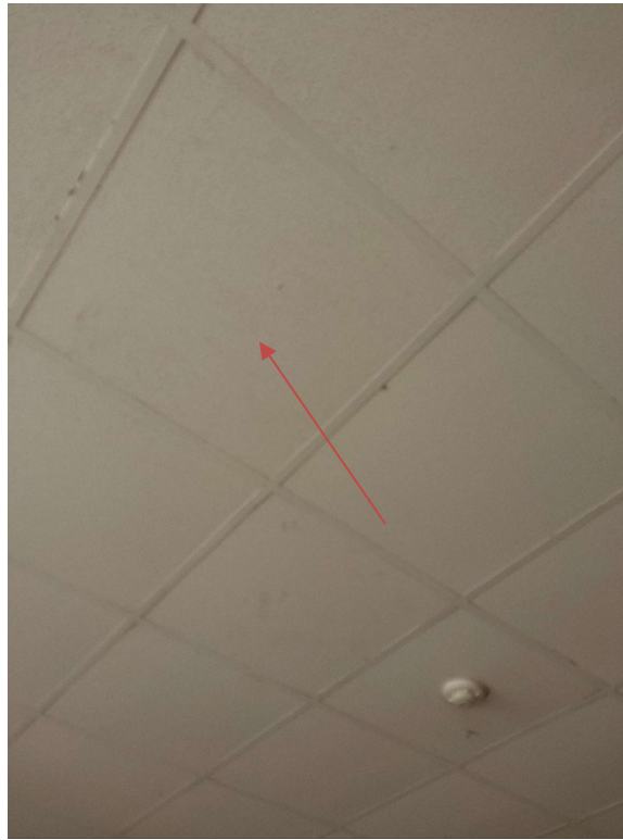
Photograph No. 7 – 2’x2’ Textured pinhole pattern ceiling tile was observed in Room 1045. The ceiling tile was sampled (S05A,B,C) and is non-asbestos.
