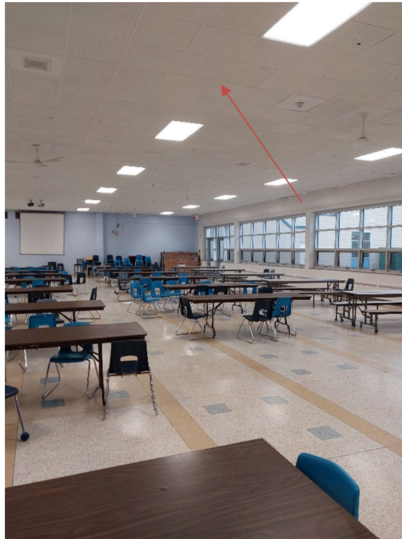
Photograph No. 9 – 2’x2’ Small fissure random pinhole pattern ceiling tiles were observed in Room 1042. The ceiling tiles were sampled (S06A,B,C) and they are non-asbestos.
