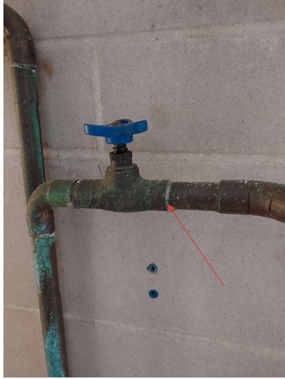
Photograph No. 13 – Suspect lead-containing solder on pipe connects was observed within Room 1044 and may also be concealed beneath building finishes.
