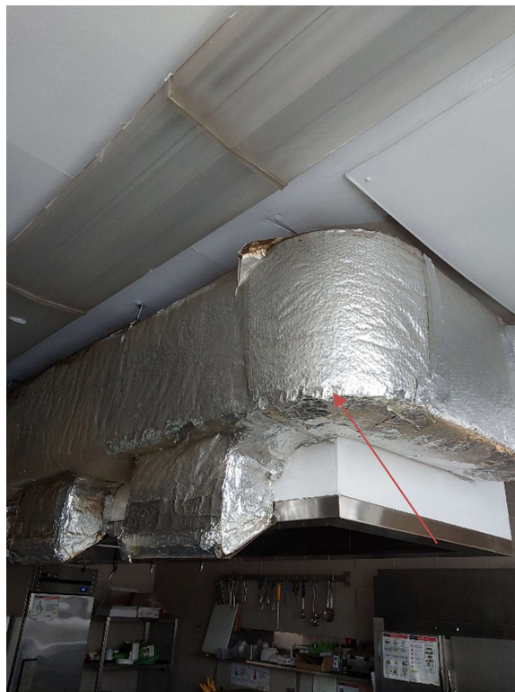
Photograph No. 10 – Foil wrapped fiberglass insulation was observed on ventilation within Room 1044A and does not contain asbestos.
