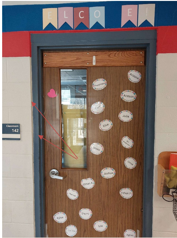
Photograph No. 1 – Sealant was observed on interior door frames. The sealant was sampled (S05A,B,C) and does not contain asbestos. Blue paint on frames observed throughout the subject area was sampled (LP03) and is confirmed low level lead-containing.
