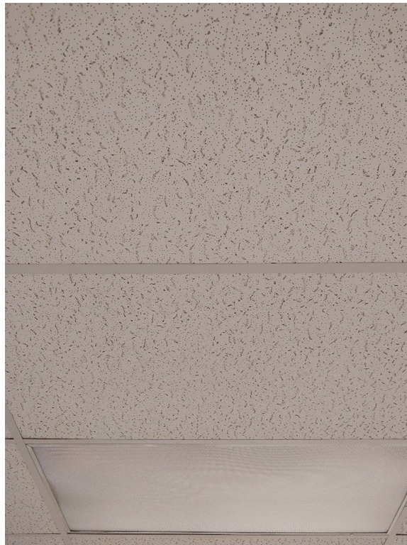
Photograph No. 10 – 2'x4' Long fissure random pinhole was observed in the academic work room 143. The ceiling tile was sampled (S04A,B,C) and does not contain asbestos.
