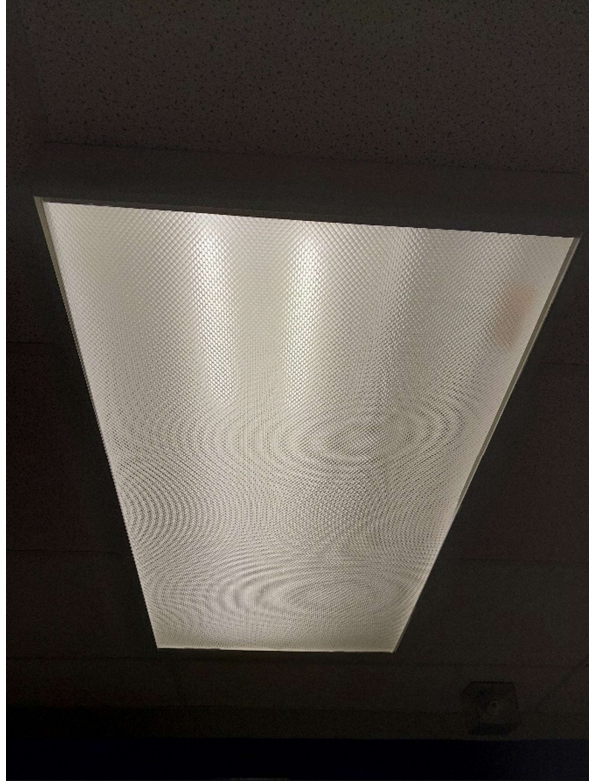
Photograph No. 5 – Mercury-containing fluorescent light tubes were observed throughout the interior. Associated light ballasts could not be inspected and may contain PCBs.
