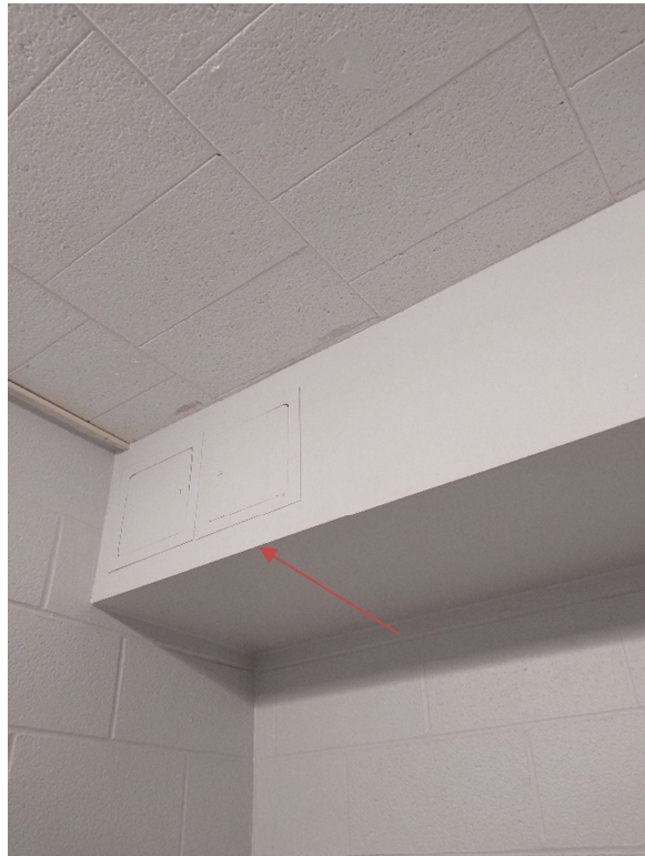
Photograph No. 6 – Drywall bulkheads were observed in the boys and girls washrooms. The drywall compound was sampled (S02A,B,C) and does not contain asbestos.
