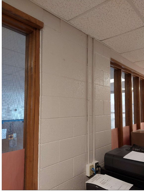
Photograph No. 7 – Concrete block mortar was observed throughout the interior and was sampled (S01A,B,C,D,E). The block mortar does not contain asbestos. The associated primer/sealant was also sampled (S03A,B,C) and does not contain asbestos.
