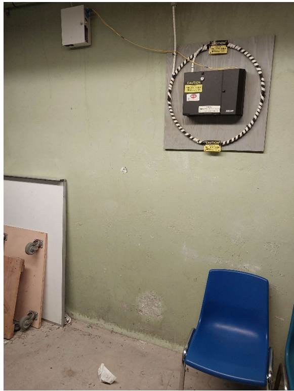
Photograph No. 8 – Green paint within the basement boiler room was sampled (LP01) and is confirmed low level lead-containing.
