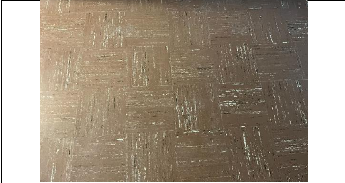
P5 – Asbestos-Containing 9"x9" Brown with Beige and Black Streak Vinyl Floor Tiles
