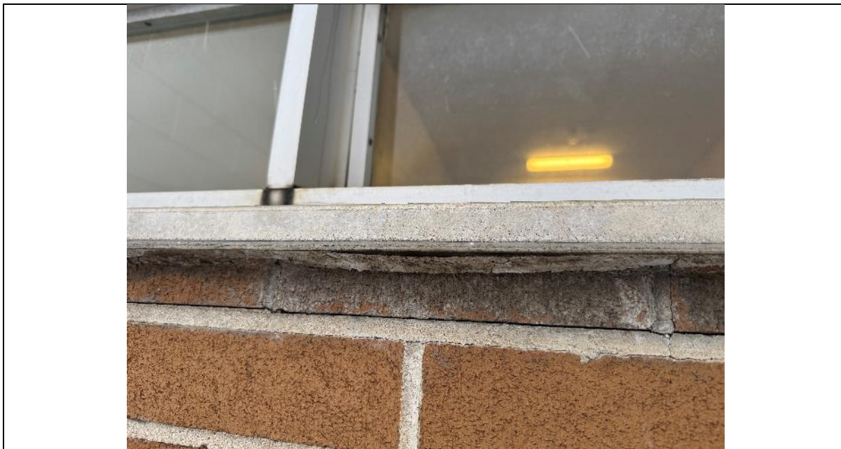
P8 – Asbestos-Containing Exterior Grey Caulking
