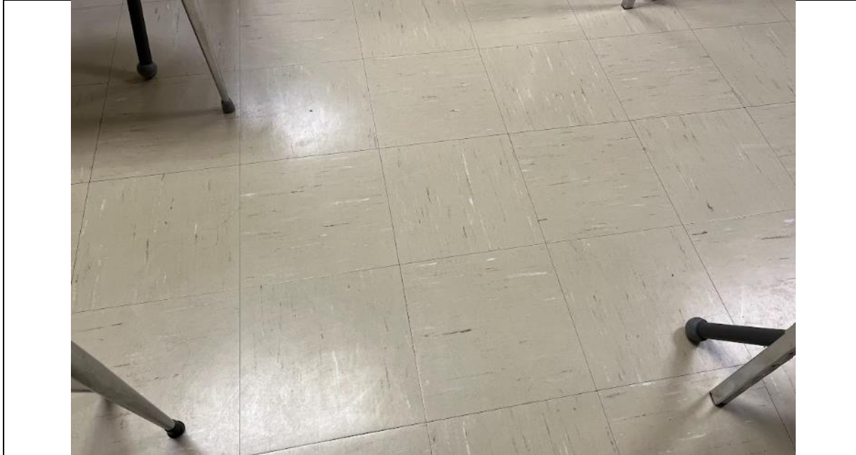
P7 – Asbestos-Containing 12"x12" Beige with Brown/White Streak Vinyl Floor Tiles
