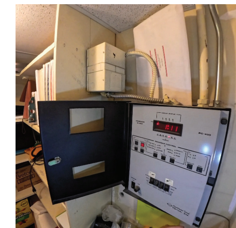
6 Existing Time Clock
