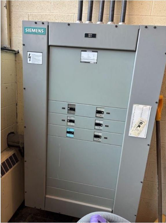
EX Switchboard HVD-B.
