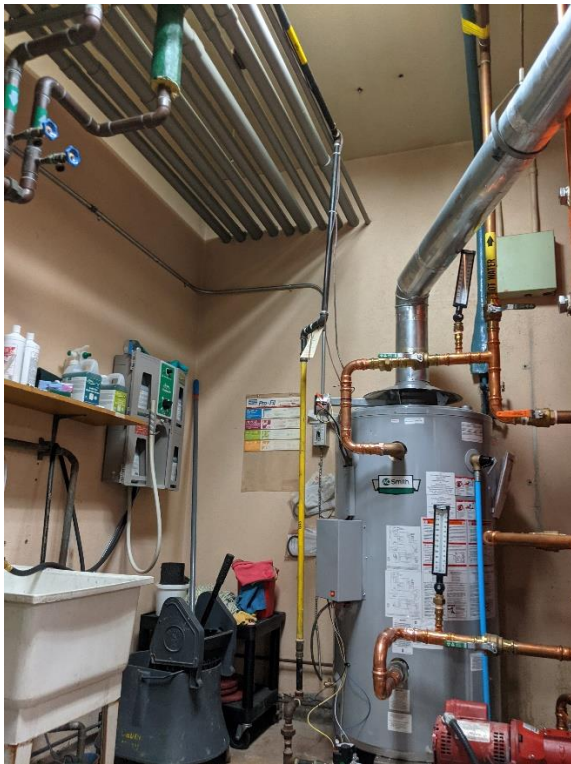
MECHANICAL ROOM B6-11
