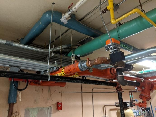
MECHANICAL ROOM B6-11
