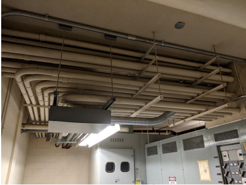
ELECTRICAL SERVICE ENTRANCE ROOM B6-12
