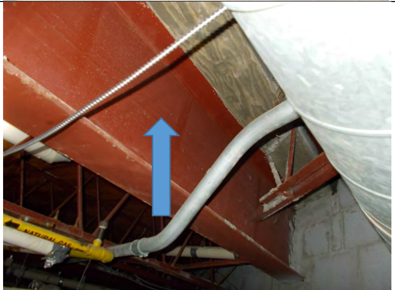
Photograph 2: View of the lead-containing red paint on the beam in the ceiling space of the library on the ground floor at the Subject Location.
