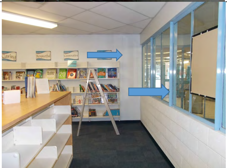
Photograph 3: View of the lead-containing white paint on block wall and light blue paint on the window frame in the library on the ground floor at the Subject Location.
