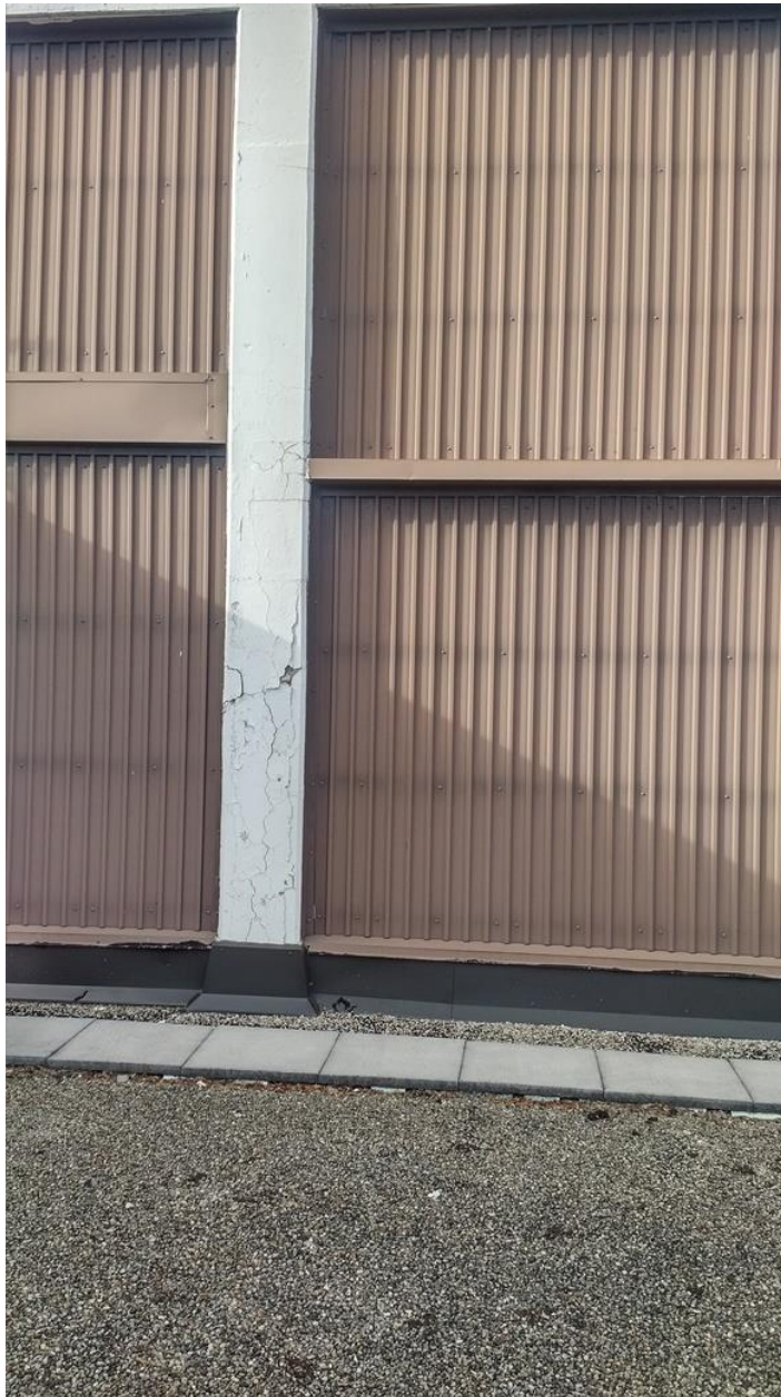
Column 1 – Remove spalled concrete, repair and paint to match existing,
