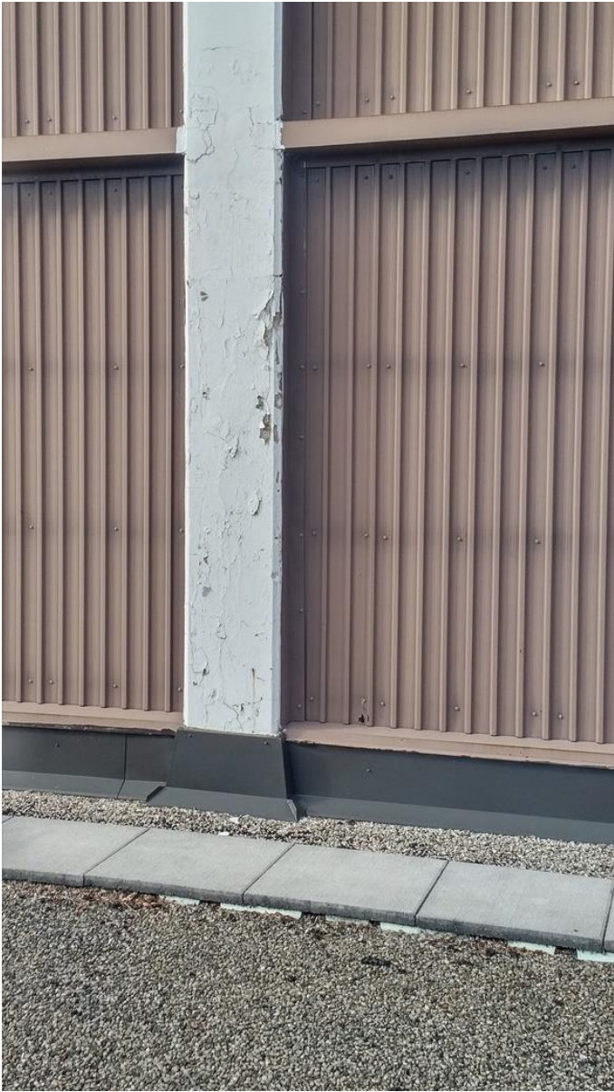
Column 2 - Remove spalled concrete, repair and paint to match existing.
