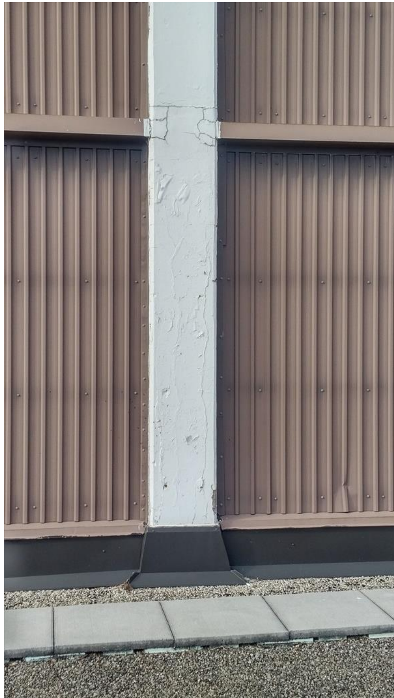
Column 3 - Remove spalled concrete, repair and paint to match existing
